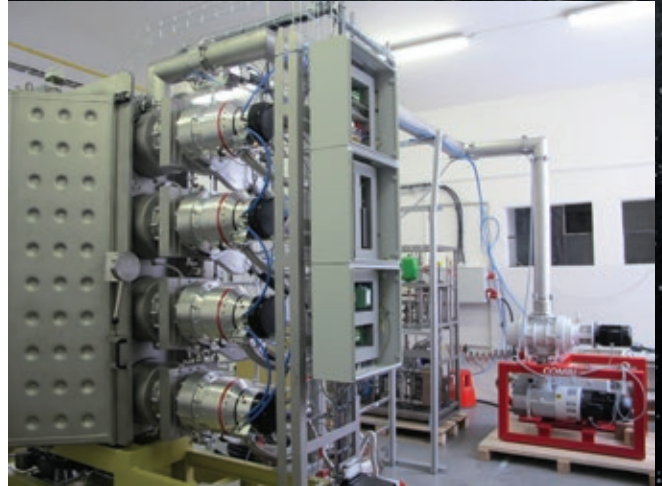
Vacuum drying system
