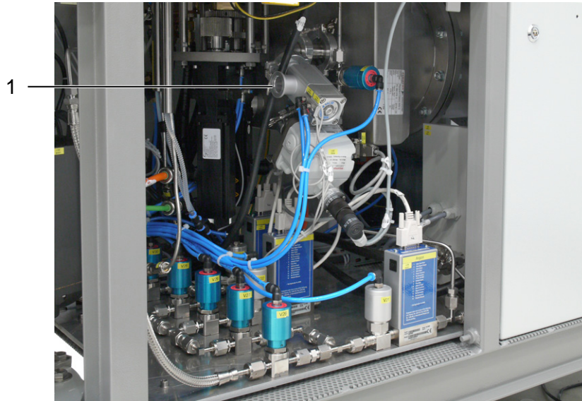
Fig. 7: Connection for venting gas on the process chamber
