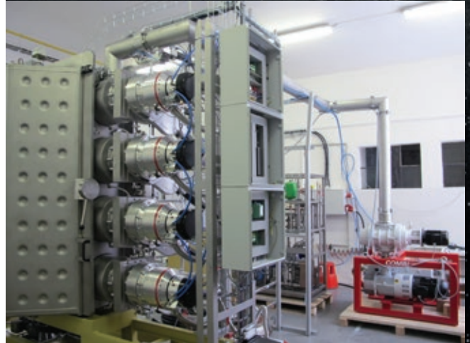
Vacuum drying system
